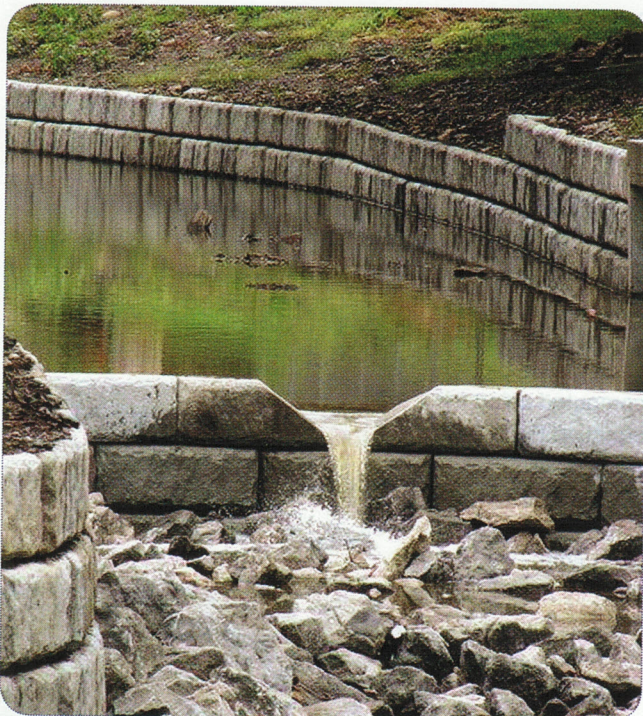
Engineers designed the walls to withstand sporadic water flows and keep off private property.
